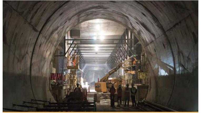
A metro line tunnel and station providing a safer and more sustainable transport system is under construction in Lima, Peru.
